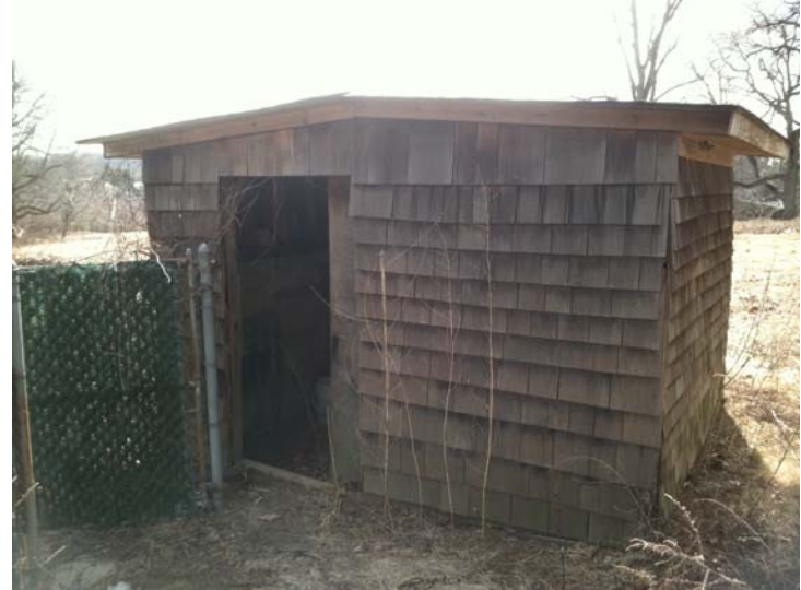
14. Looking southwest at pool equipment house
